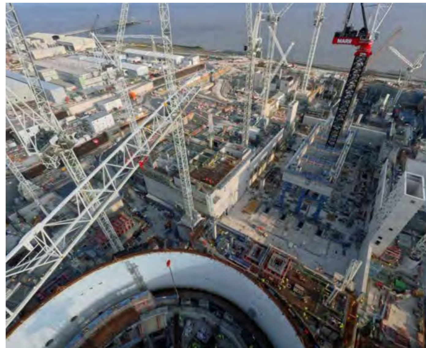
HPC Construction site with views to the Bristol Channel. Photo courtesy of EDF Energy
